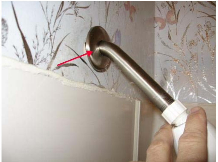
Shower pipe loose at wall intersect, 2nd flr bath
