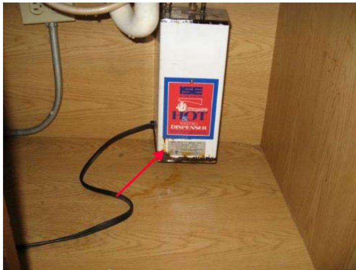
Hot shot water heater not functional
