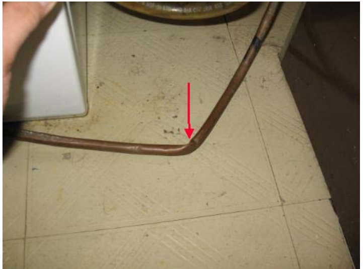
Humidifier drain kinked
