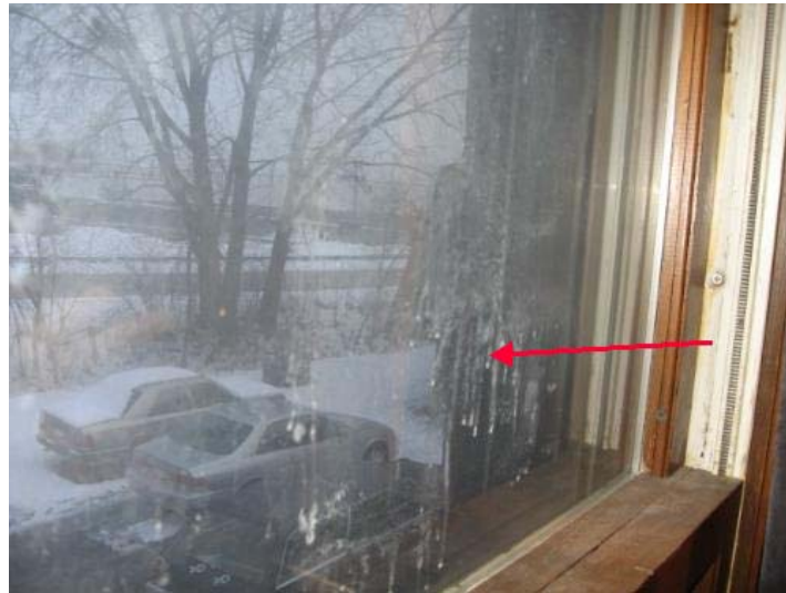
Fogging btwn window panes, thermal seal break suspected
