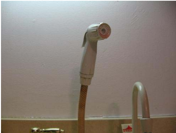
Kitchen spray diverter has active leak
