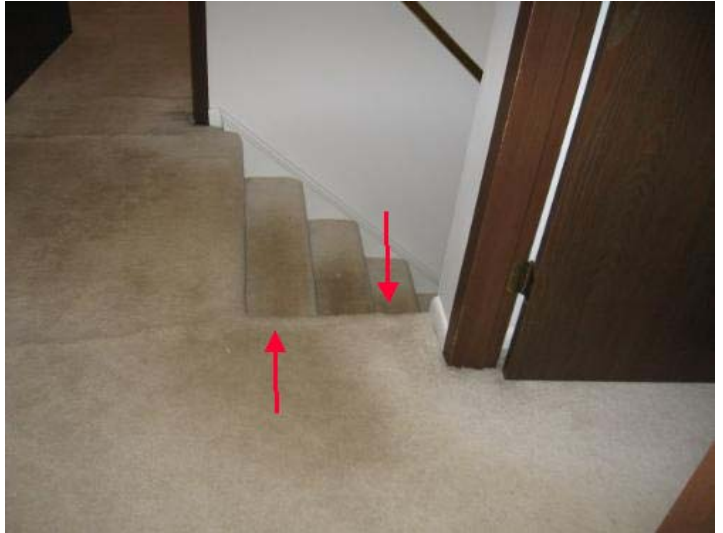
Safety rail omitted on 2nd flr
