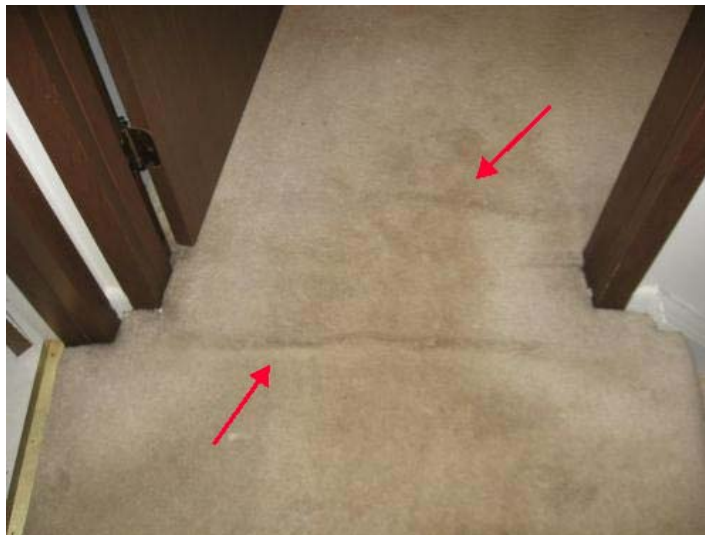
buckling carpet on 2nd flr, trip hazard
