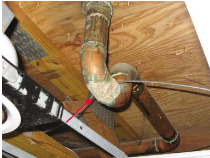
Corrosion on drain line (basement view)
