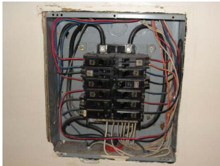
View of service panel
