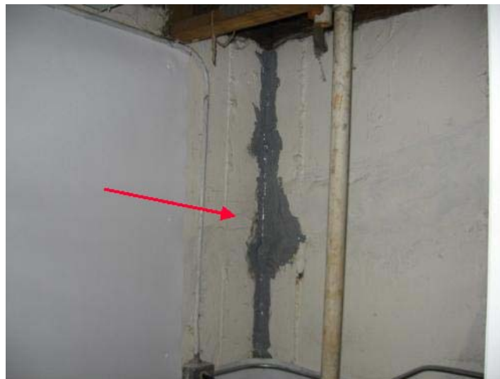
Previous foundation repairs noted
