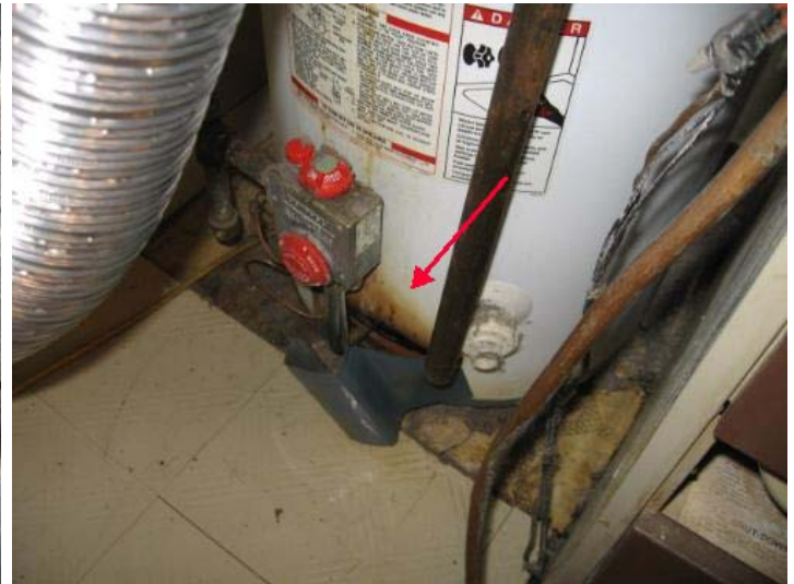
Evidence of flame rollout
