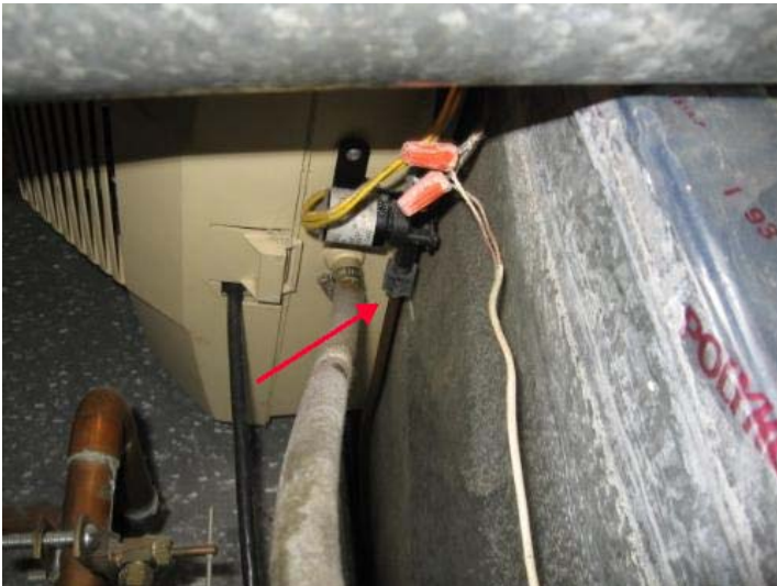
Humidifier leak noted
