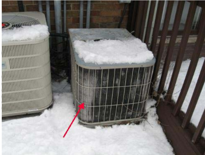
View of AC condenser, bent fins noted
