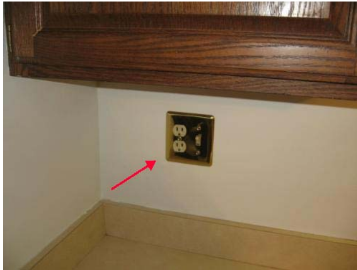
GFCI outlet needed over counter in kitchen
