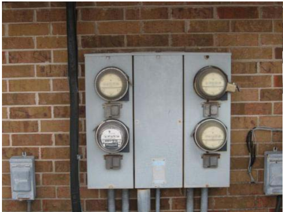
View of electrical meters 100amp
