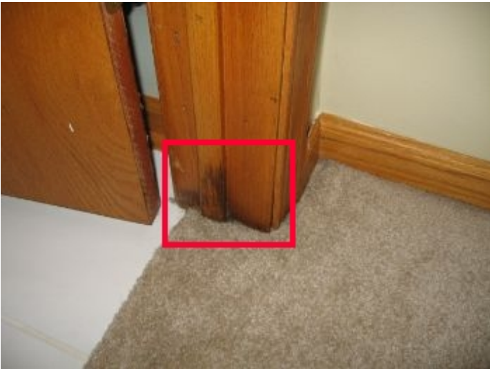
Evidence of water damage on interior door jamb of basement bathroom door; undetermined source of penetration; no other evidence of water stains or penetration noted; monitor area for any signs of water penetration
