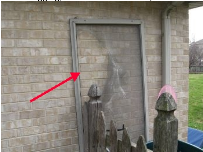
Rear sliding screen doors are removed, door frames are present outside both with torn screens; repair as needed, install and reevaluate
