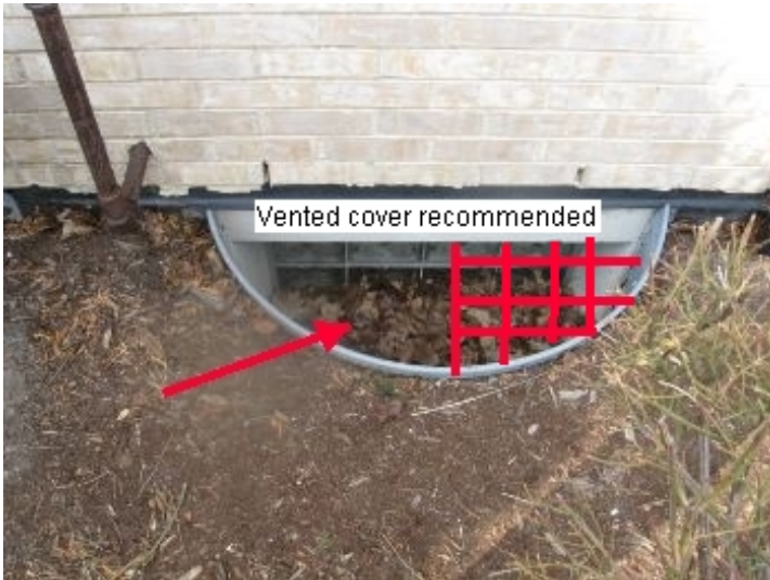
Basement window wells are full of leaves and debris, clean as needed : Well covers recommended
