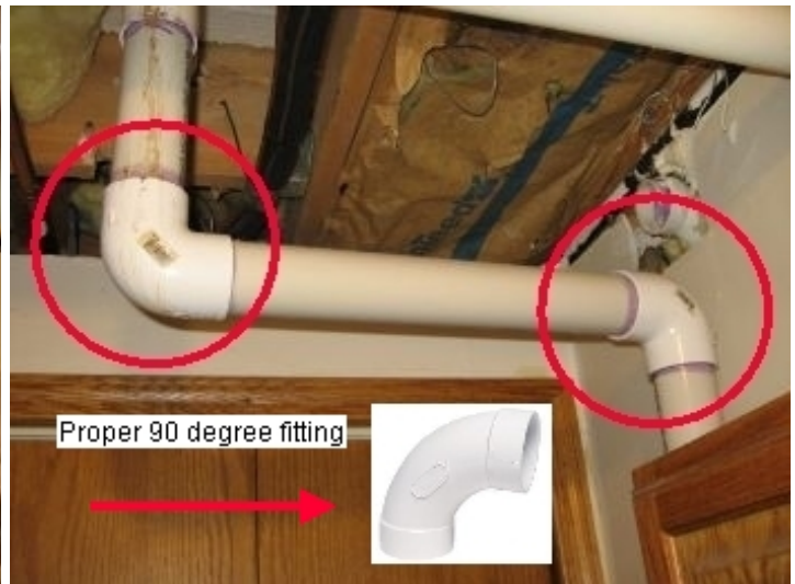
Ejector discharge line has improper short 90 degree joints installed; all 90 degree joints should be longer sweeping joints to ensure against clogging and ensure functional water flow. Consult a licensed plumber for evaluation
