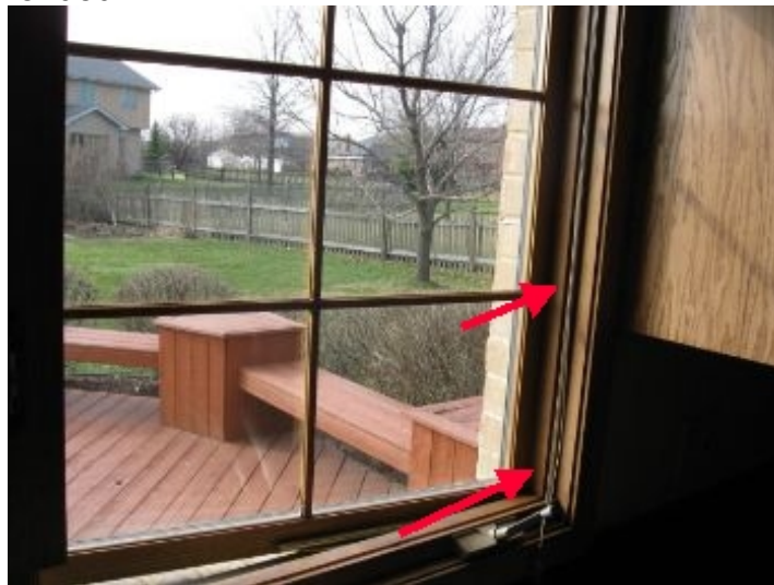
Kitchen window over the sink does not open completely, window sash hits style; adjust/repair as needed
