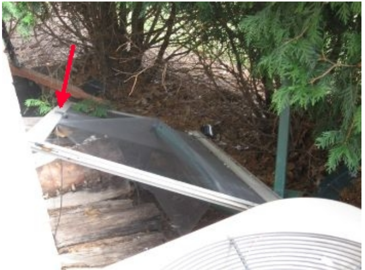
Rear sliding screen doors are removed, door frames are present outside both with torn screens; repair as needed, install and reevaluate
