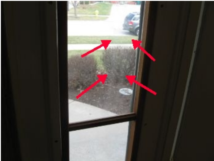
Front entry door side light to north has minor hazing between glass, may be indicative of a thermal seal break; monitor condition for further fogging, or moisture between panes
