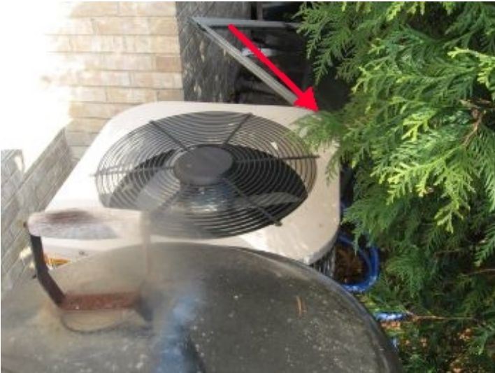
Large shrub in close proximity to condensing unit; this will restrict air flow to unit which reduces efficiency of unit and may reduce life expectancy of unit
