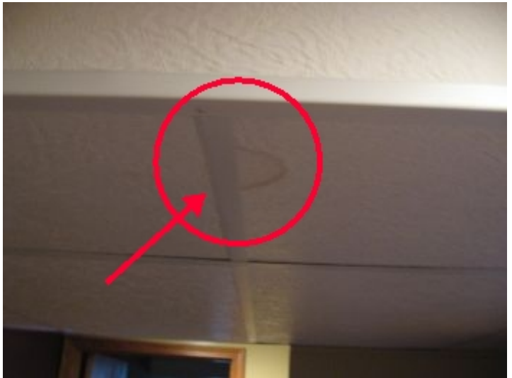
Small area of water stains noted on drop ceiling tiles, further inspection revealed the main water supply line overhead; no leak detected stains may be result of pipe sweating during periods of high humidity. Recommend application of pipe insulation to prevent sweating.
