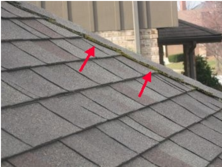
Minor moss build up noted on shingle edges
