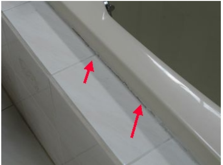
Deteriorated caulk noted on jacuzzi tub perimeter, new application recommended to prevent water seepage
