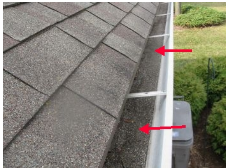
Evidence of shingle granule loss noted in gutters
