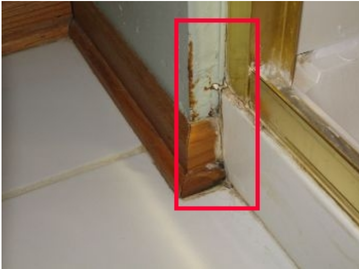
Basement bath shower base perimeter has areas of water penetration beyond shower walls and doors; may be result of deficient caulk application
