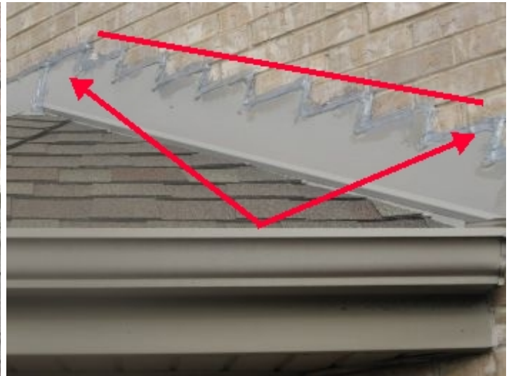
Evidence of recently applied caulking on rear flashing over kitchen dinette doorway; unk if new application was due to leaking or merely a maintenance precaution
