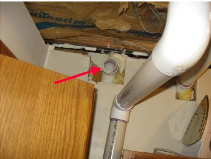
Ejector discharge line has improper short 90 degree joints installed; all 90 degree joints should be longer sweeping joints to ensure against clogging and ensure functional water flow. Consult a licensed plumber for evaluation
