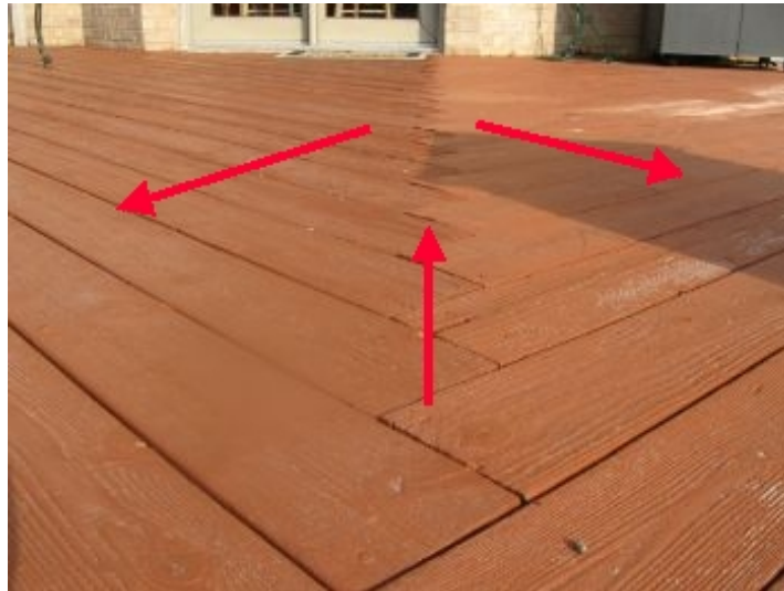
Evidence of deck settlement at perimeter; no view of footings or support posts for proper evaluation
